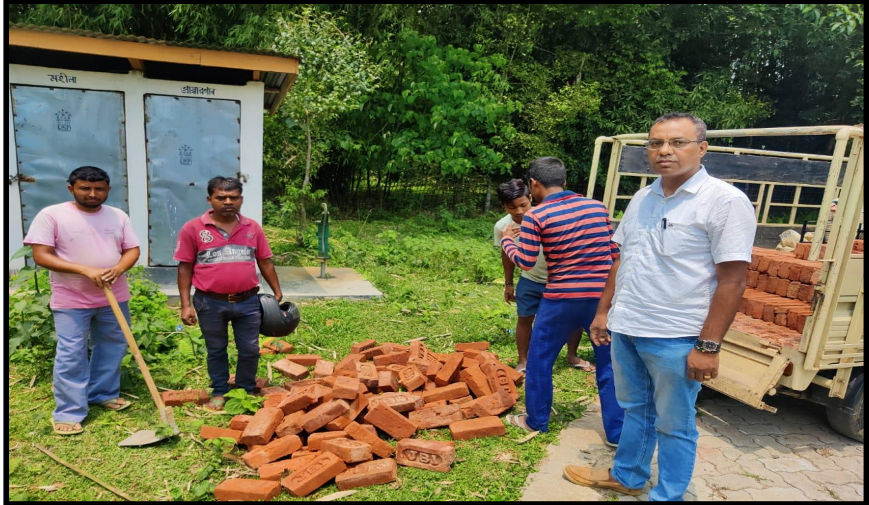
Photo: Supply of materials for construction of Dustbin under Green and Clean Campaign of College, 21-05-2022
