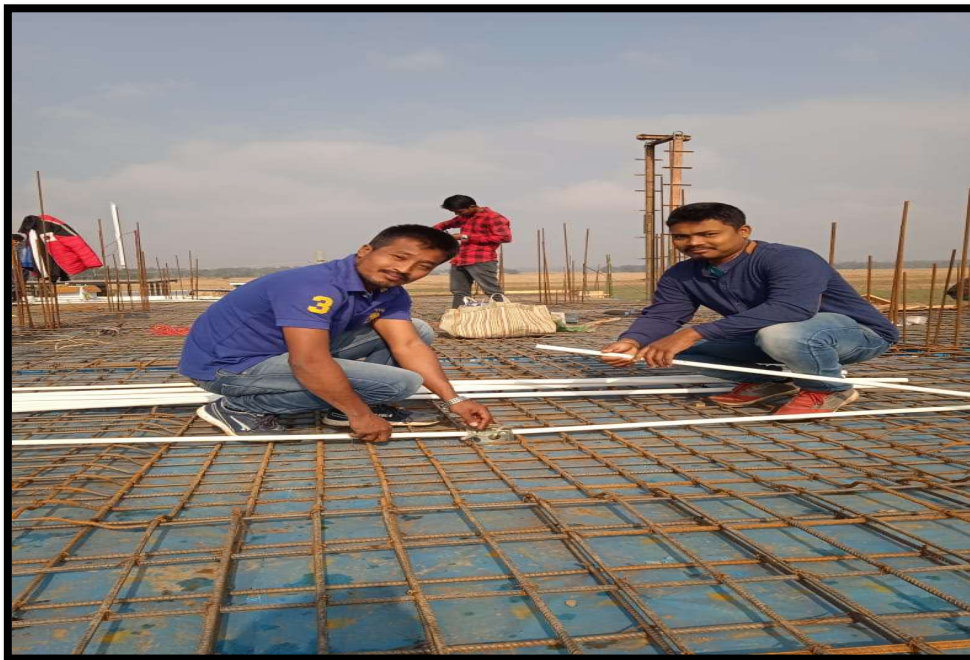
Fig. Mr. Satyajit Saikia and Mr. Pranjal Saikia, Professional Electrician (Batch: 2017-19) while doing Domestic Conceal Wiring
