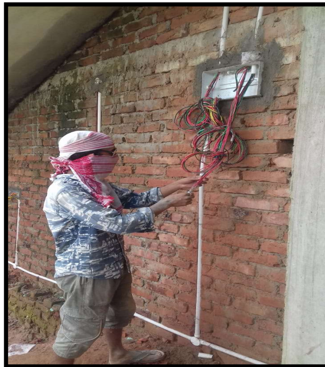
Fig. Mr. Bhaskar Senapati, Professional Electrician, (Batch: 2017-19) while doing Domestic Conceal Wiring
